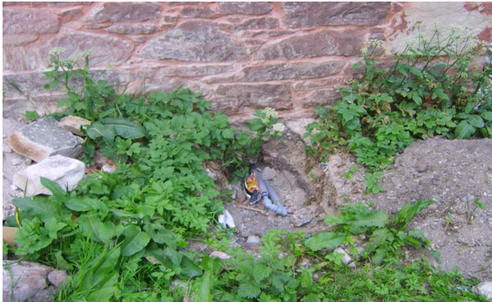
Photograph No 4 Pipes Through / Under Building Foundation
